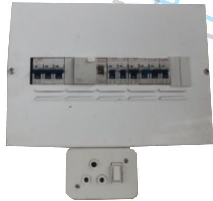
3 Phase 30amp Distribution Board (DB)
