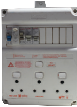
Single Phase 30amp Distribution Board (DB)
