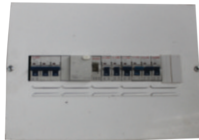
3 Phase 60amp Distribution Board (DB)
